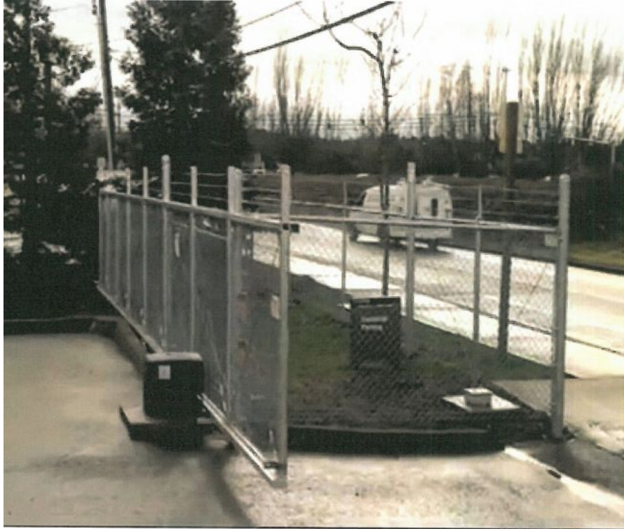
Example of automatic gate/fence (without windscreen)
